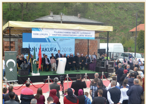
Laying of the stone foundation for construction of the Waqf's administrative center "Madrasa" in Fojnica
